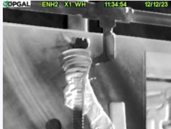
Pneumatic controller leak
