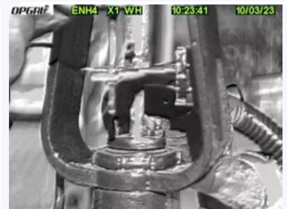
Valve stem packing leak
