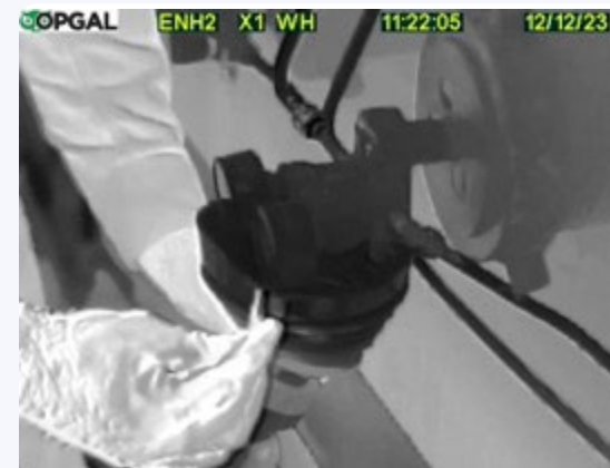
Pneumatic valve leak
